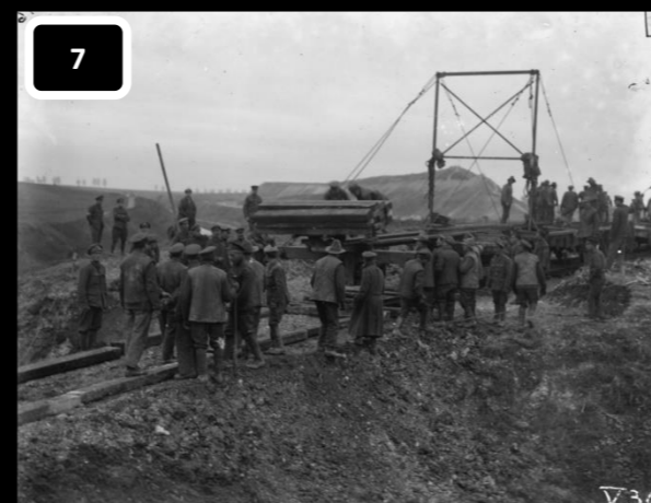
IWM / Q 47113 / Achiet-Marcoing Line (Hermies Diversion). C. O. R. C. Track-Layer handling sleepers. 22. 11. 17.
