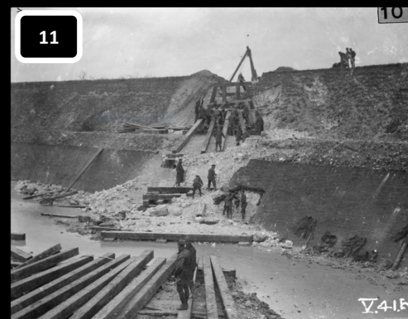
IWM / Q 47168 / Achiet-Marcoing Line (Hermies Diversion). Trestle bridge carrying line over Nord Canal in course of construction. 27. 11. 17. Map Ref. Sheet 57C. K. 26C.
